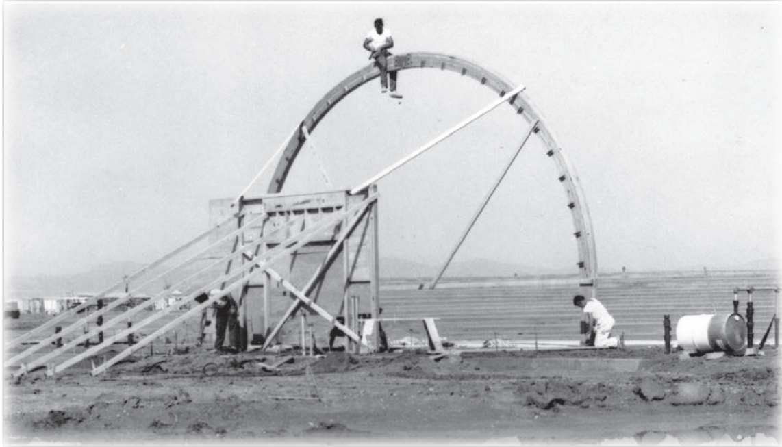
Construction of the Sun Bowl outdoor amphitheater located at 107th Avenue and Clair Drive in Sun City began in 1965. The facility officially opened in 1966. Over the years, the venue has hosted some of the biggest names in the entertainment world, as well as local events, celebrations and festivals.
