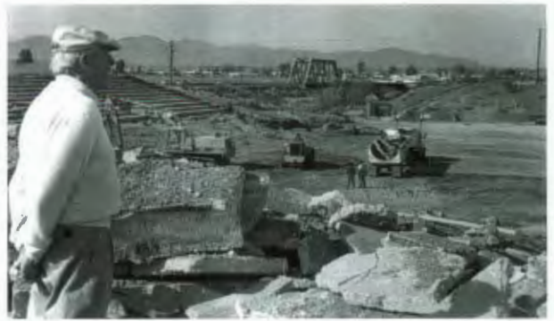
The stadium gave way to The Fountains at Sun City, an apartment complex.
