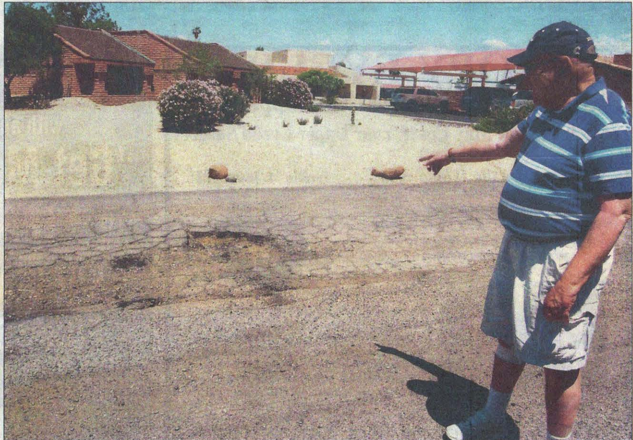
Charlie Schill points to the deepest of the potholes in the alley behind his home south of Coggins Drive at 105th Avenue. His homeowners association pays to maintain half the alley but the other half is left to deteriorate because no one is claiming ownership. [Independent Newsmedia/Rusty Bradshaw]
