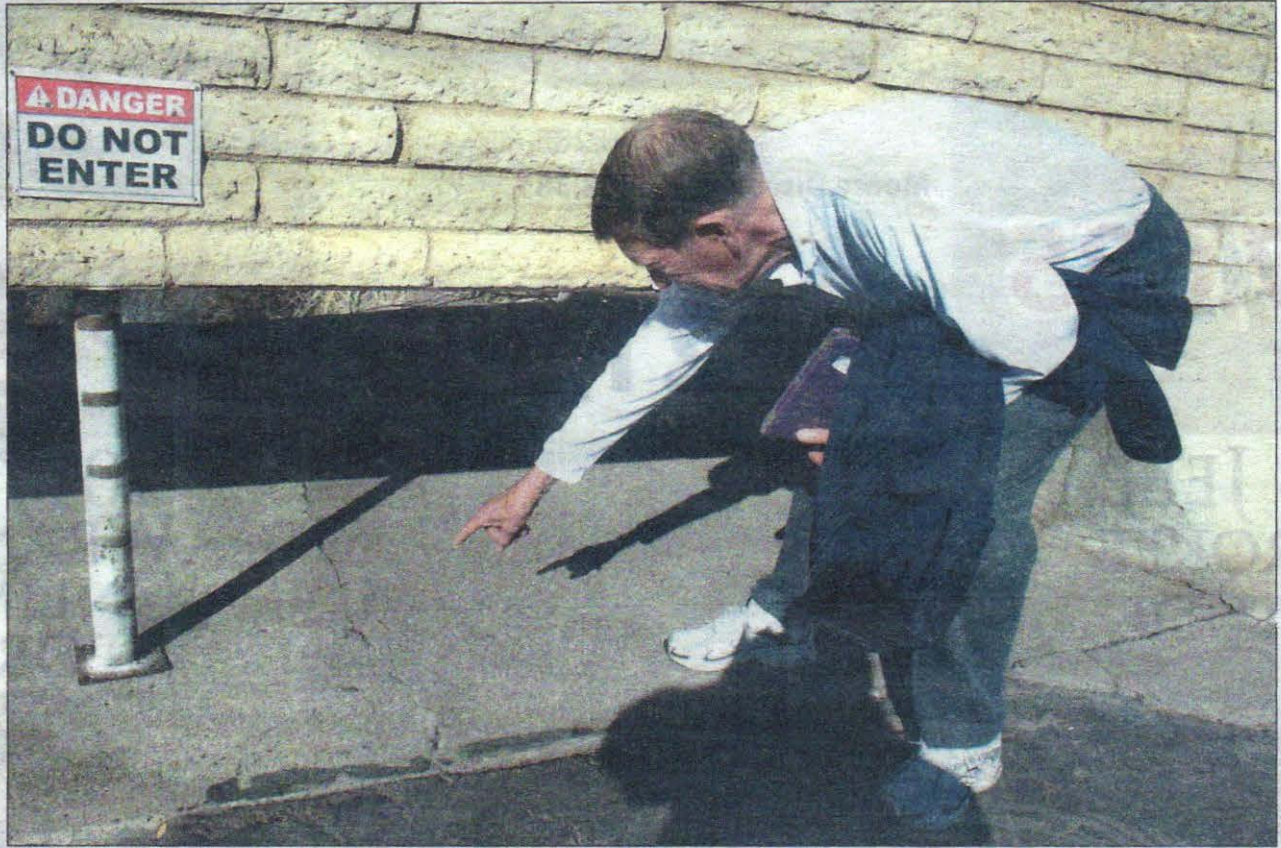
Sun City resident Tom Taylor points out a crack in the concrete drainage port for water runoff behind his condo and under a portion of the community wall. Mr. Taylor and other residents are concerned the crack could eventually bring down the wall. [Rusty Bradshaw/Independent Newsmedia]
