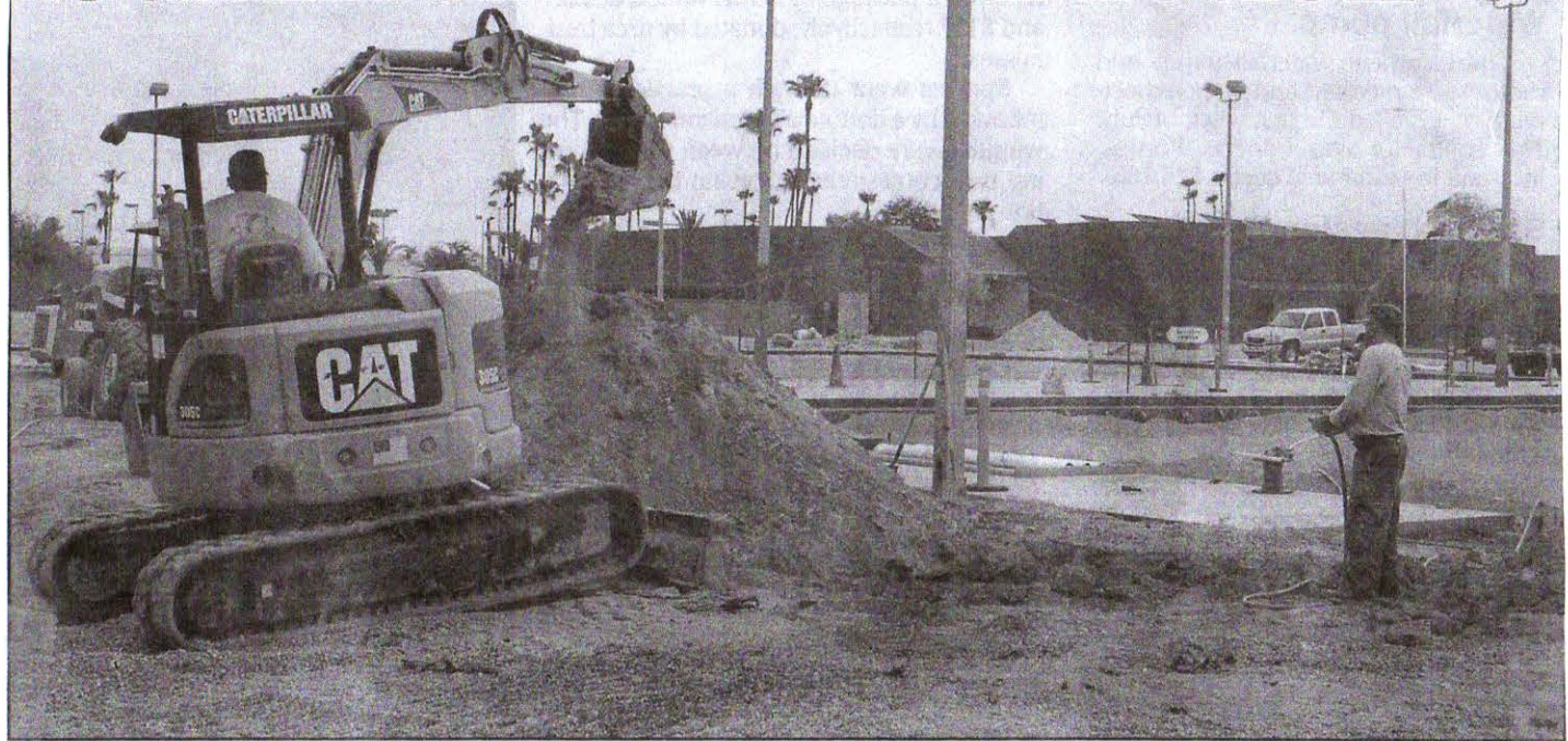
Workers dig a trench as part of the total renovation of Bell Recreation Center, 16820 N. 99th Ave., lawn bowl greens. It is one of several major construction and renovation projects at various Recreation Centers of Sun City facilities this year.
