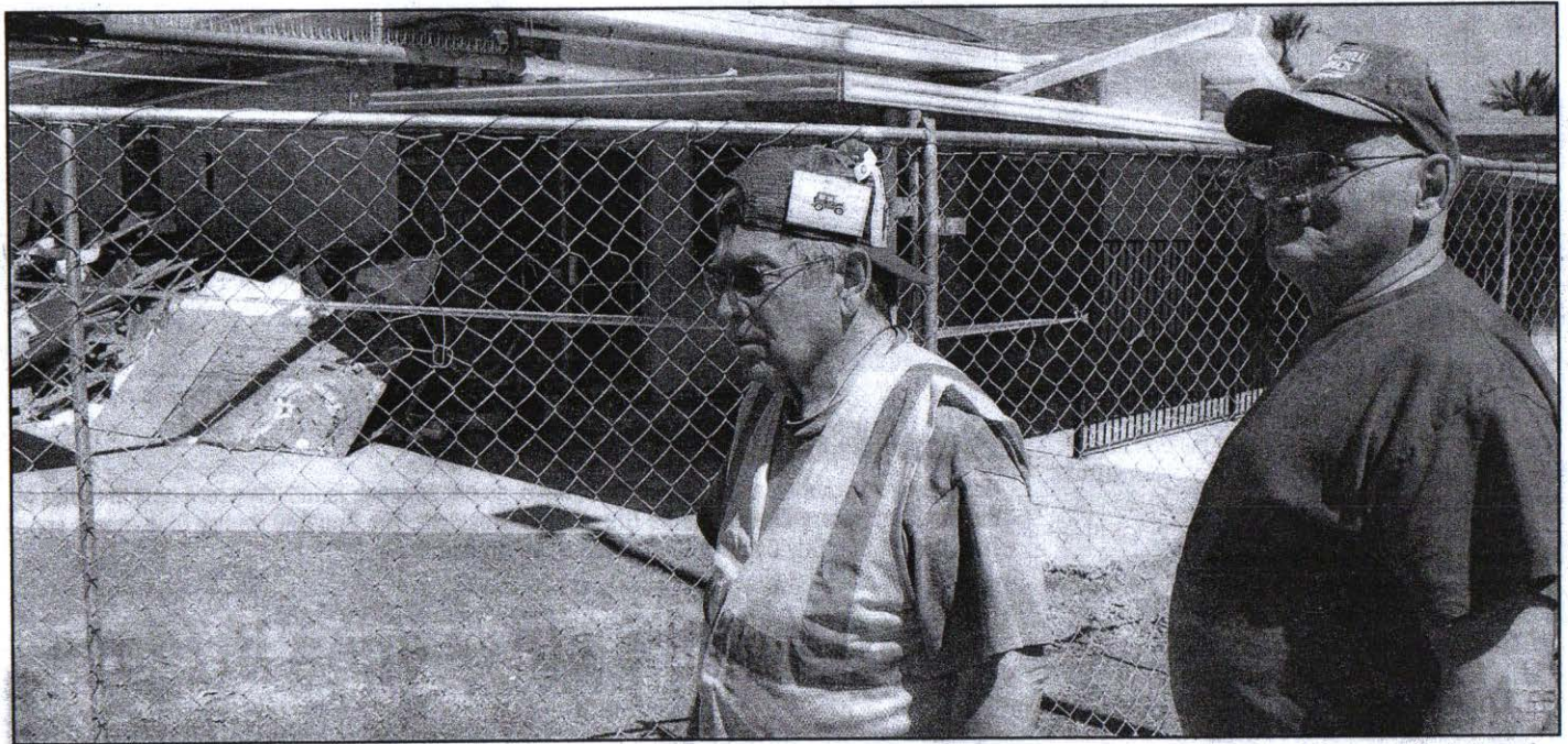
Independent Newspapers/Rusty Bradshaw Frank Hogan, left, and Lyle DeRose look over the asbestos abatement work at Fairway Recreation Centers, 10600 W. Peoria Ave. The remaining older portions of the center are scheduled to be demolished beginning July 5 to make way for the construction of phase two of the new Fairway Center.
