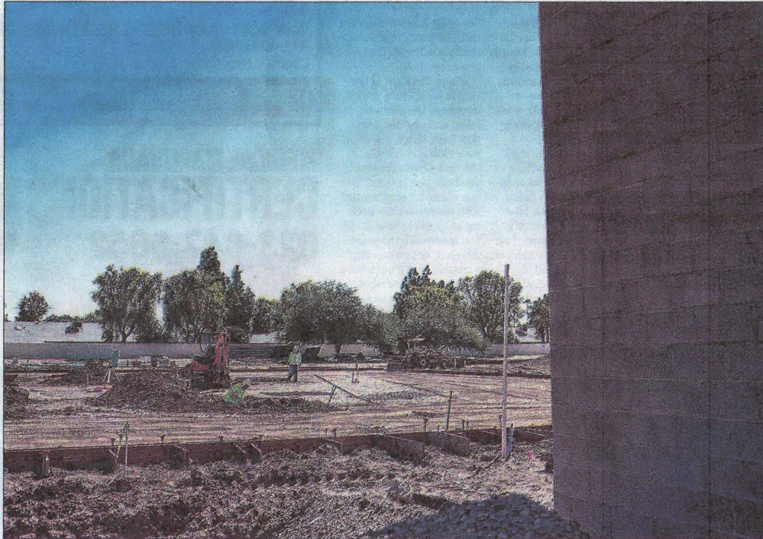
Construction continues on the future pickleball courts at Marinette Recreation Center in Sun City. (Jarod Opperman/Daily News-Sun)
