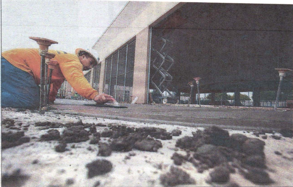
A worker smooths concrete Thursday for the sidewalk outside Marinette Center's new covered pickleball facility. [David Jolkovski/Daily News-Sun]
