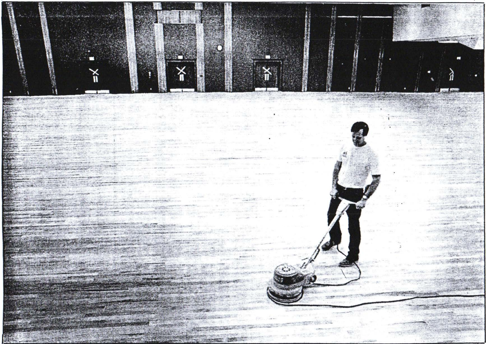
LAST TOUCHES — Jerry Scott, from Mission Hardwood in Scottsdale, works on buffing the new 17,331-square-foot oak floor in the auditorium at Sundial Recreation Center on Monday.
