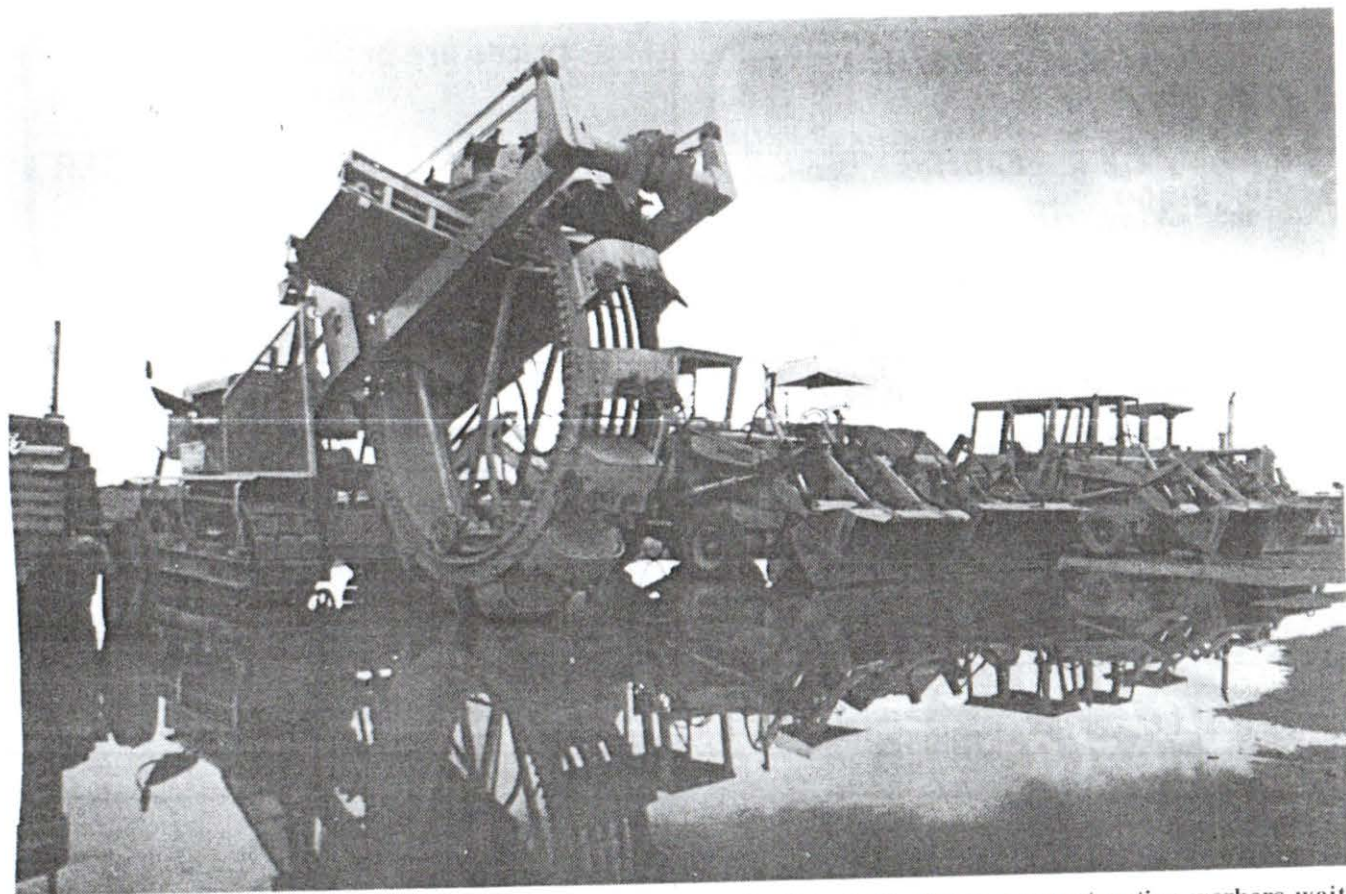
Bogged down, Del E. Webb construction equipment stands in huge puddle of water near 99th Avenue just north of Santa Fe Drive as construction workers wait for weather to clear before resuming work.
