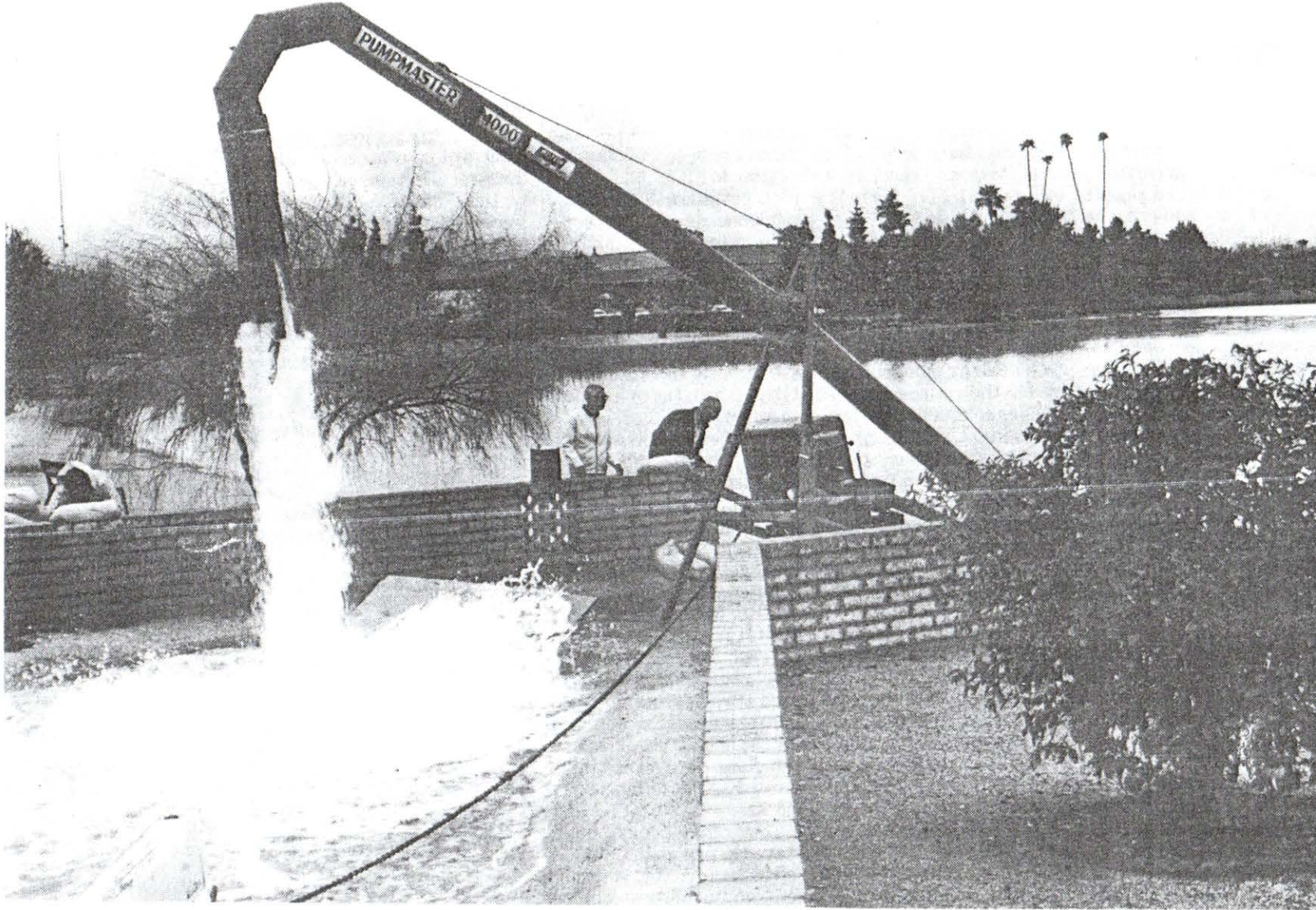
Del E. Webb Development Co. water pump removed 6000 gallons per minute from Viewpoint Lake at 103rd and Thunderbird Thursday afternoon. Lake was in danger of overflowing, so this effort was launched in order to drain water out toward New River.
