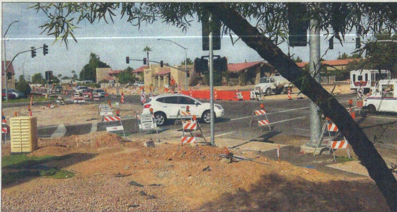
Construction work was stopped through the end of October at the Union Hills Drive and 99th Avenue intersection while utility conflicts were resolved. The work stoppage delayed completion of the project, which has caused some frustration by drivers and businesses in the area.
