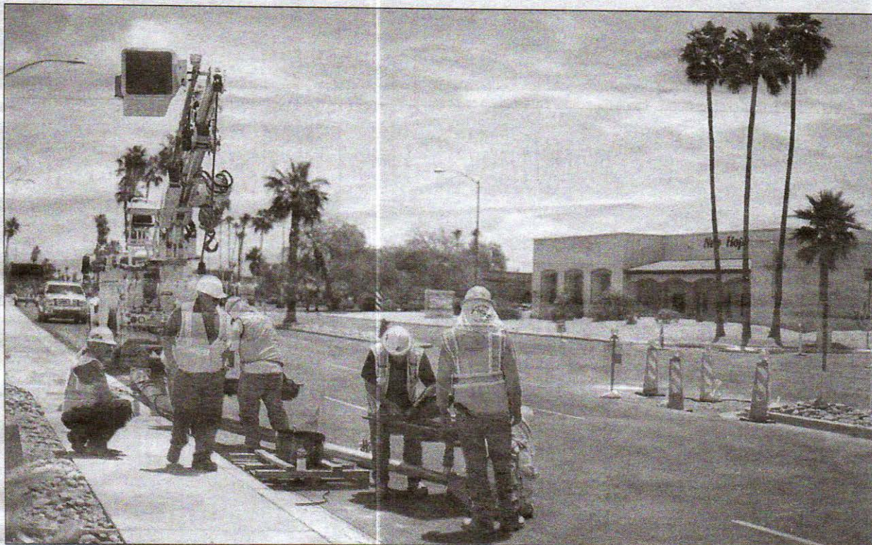
Construction crews install a "High-Intensity Activated Crosswalk," also known as HAWK, Tuesday afternoon outside the R.H. Johnson Recreation Center. The HAWK, resembling a beacon much like a traffic signal, stops traffic only when it's necessary for pedestrians to cross the roadway. [Jarod Opperman/Daily News-Sun]
