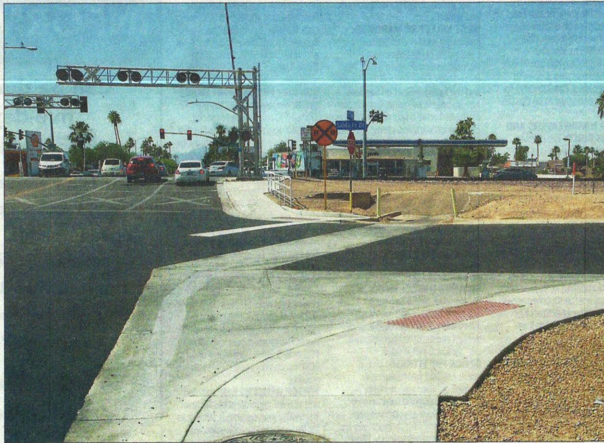
Maricopa County Department of Transportation crews recently made roadway repairs near 103rd Avenue and Santa Fe Drive in Sun City, thanks to collaboration between that organization, the Sun City Homeowners Association and a private property owner. [Submitted photo]
