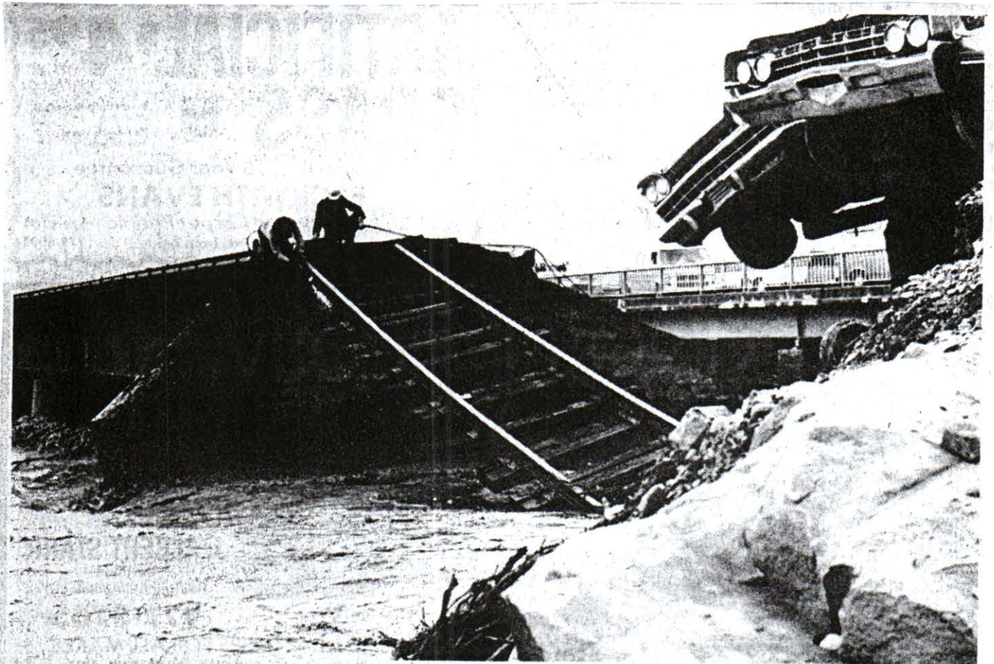
Workmen sever ties to let sagging track fall into water. First attempts at filling gap with cars failed when they floated away instead of sinking. Later, when track was
