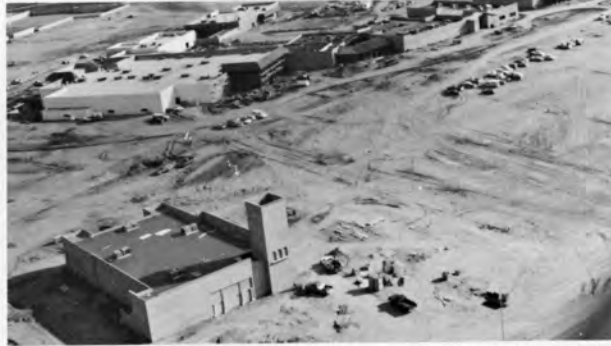
JANUARY 1979 — Johnson Rec Center, Arizona's largest private facility for recreational and creative activities, moves toward a second-quarter 1979 opening. The center's 40,000-volume library is in the foreground.
