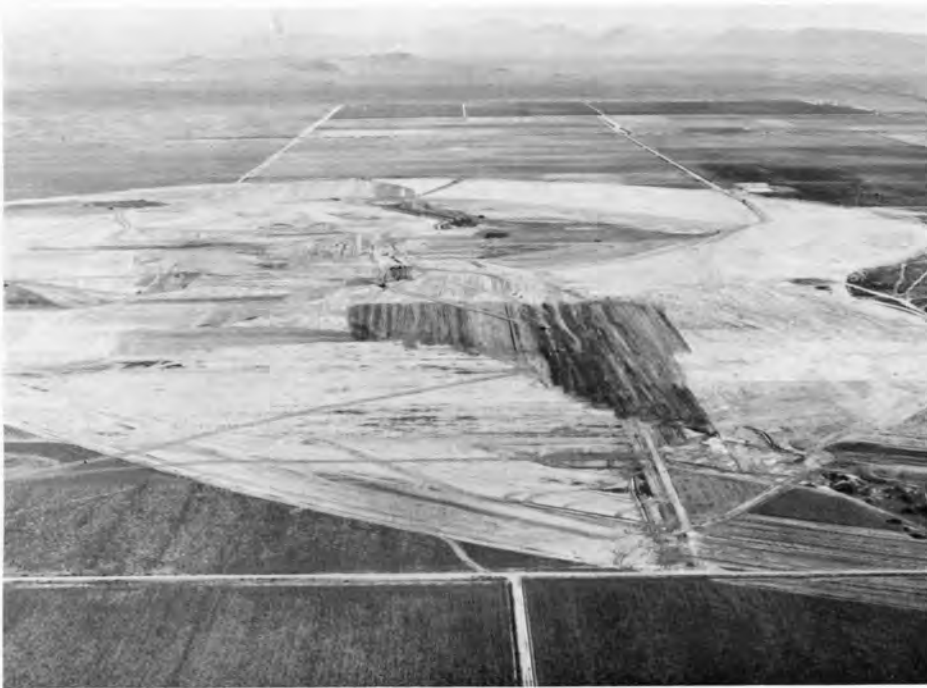
APRIL 1978 — Sun City West site development begins with graders leveling the land.
