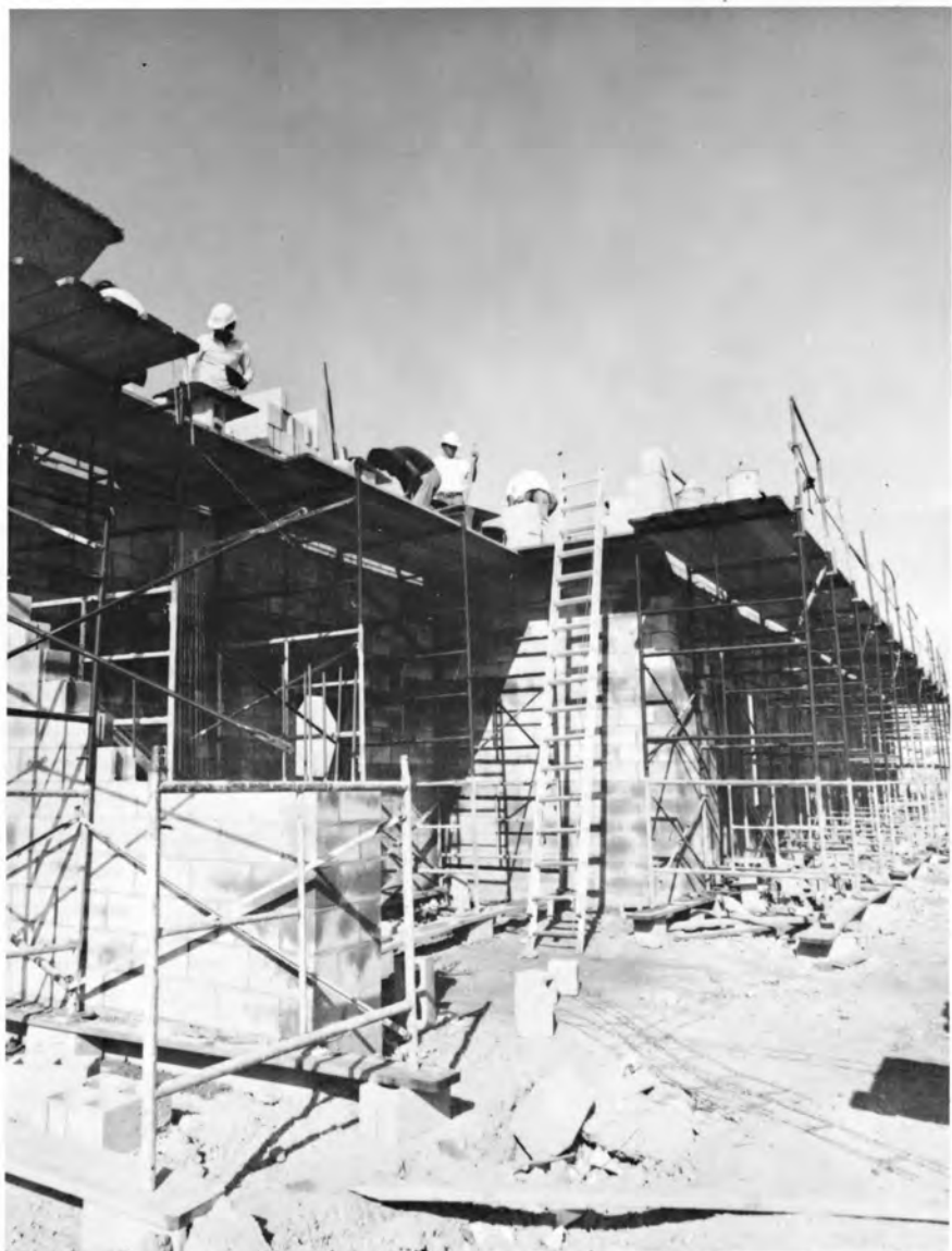
JUNE 1978 — Standing on scaffold supports, brick masons build the exterior walls of Crestview. The masons are among some 1,000 Development Company field personnel.
