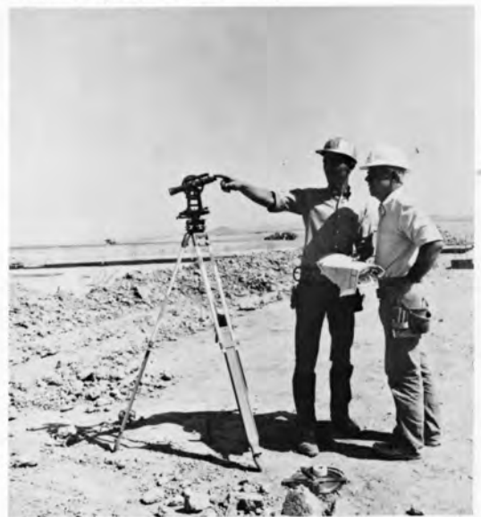
MAY 1978 — Surveyors gaze past their transit during the initial stages of construction of Crestview Restaurant.
