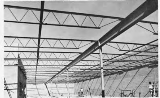
NOVEMBER 1978 — Construction continues on the crafts and ceramics rooms of Johnson Rec Center as steel I-beam girders and roof trusses are erected.
