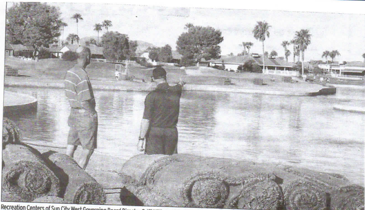
Recreation Centers of Sun City West Governing Board Director Griff Williams, left, listens as Rec Centers' Environmental Services Manager Todd Patty talks about the ongoing project at Lake No. 4 on Echo Mesa Golf Course. The lake recently received a block wall barrier that will help eliminate water loss, and workers are laying sod around the lake border. Echo Mesa is expected to reopen for play on Oct. 15. [Submitted photo]
