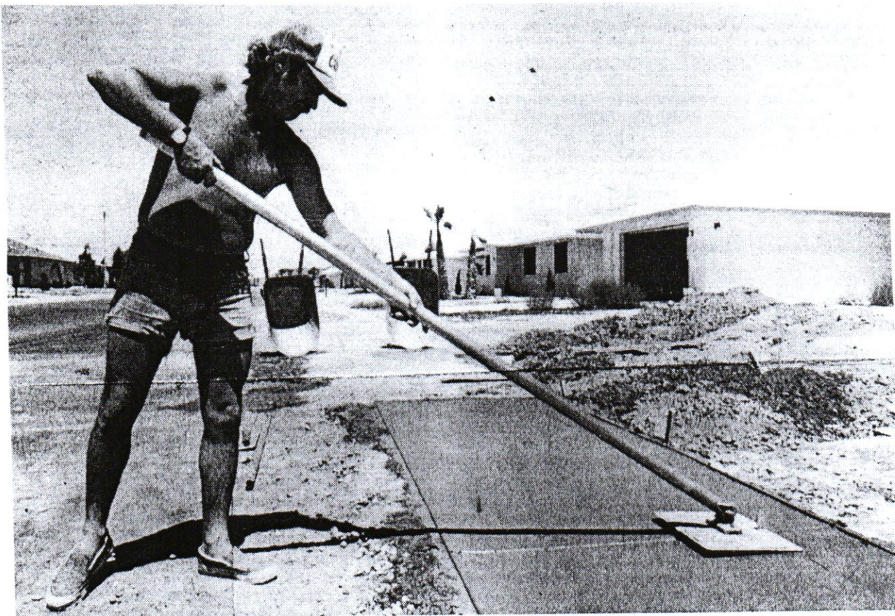
Lynn Clements finishes the concrete of a sidewalk in front of a new Sun City West home. (News-Sun photo by Jim Painter)
